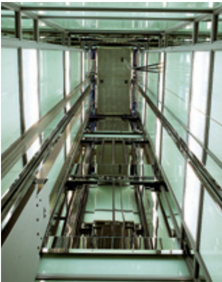
Lödige: lifts and escalators with state-of-the-art technology
