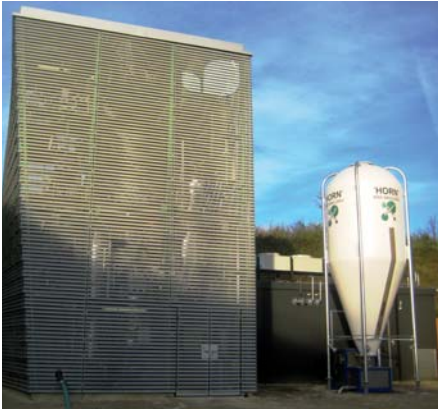
Wood gasifier installation
